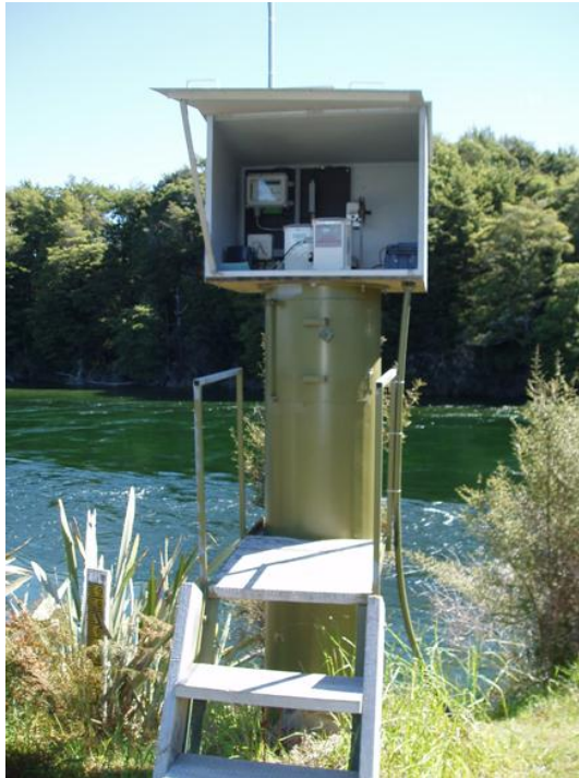
Figure 13 – Typical Stilling Well Housing design
