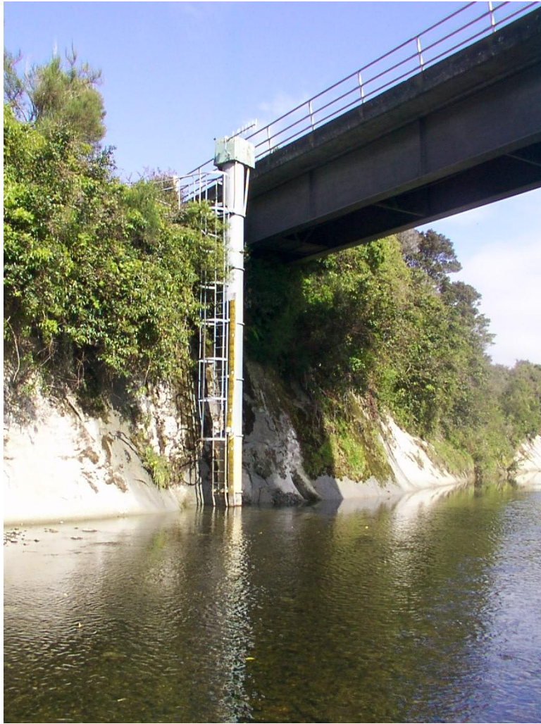
Figure 12 – Water Level Station Showing Multiple Sections and Housing
