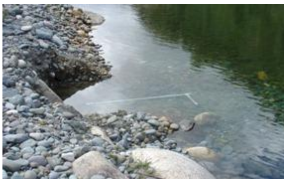
Figure 11 – Example of Intake and Static Pipe
